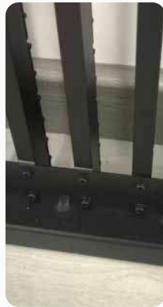
Rear maintenance module
